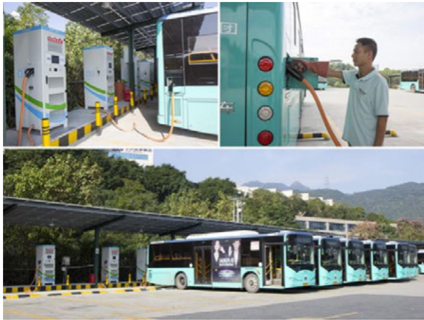
Figure 6-7 Liuyue charging station operated by Winline
